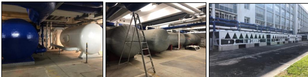
Phase II installation of Tygerberg campus's central HVAC system (from left): the central chiller plant, buffer tanks and water storage tanks.
